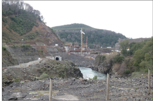
The Angostura Hydroelectric Plant
