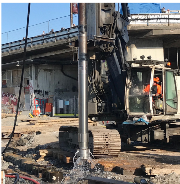
Drilling with Wassaras water-powered hammer gives a nice and clean work environment
